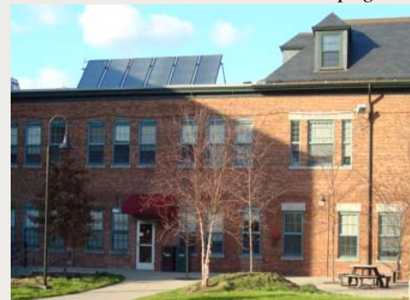
Solar thermal panels on top of Blackstone North
