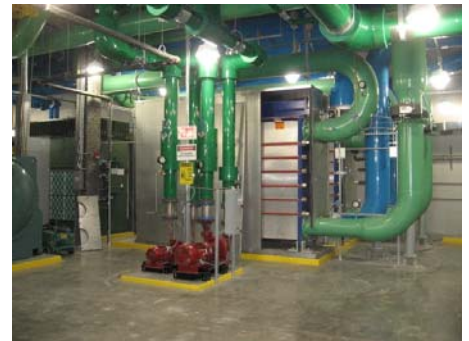
E&U's Free Cooling Heat Exchanger
