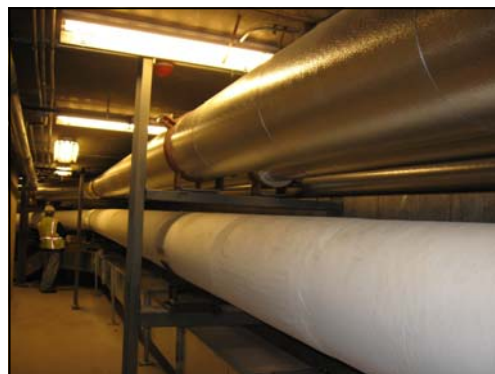
Hundreds of feet of steam pipe connect the WCC to Harvard's District Heating System
