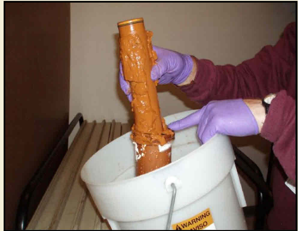
Iron sludge from a blocked strainer
