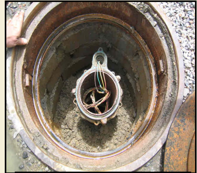
Open Well Head – Standing Column Well
