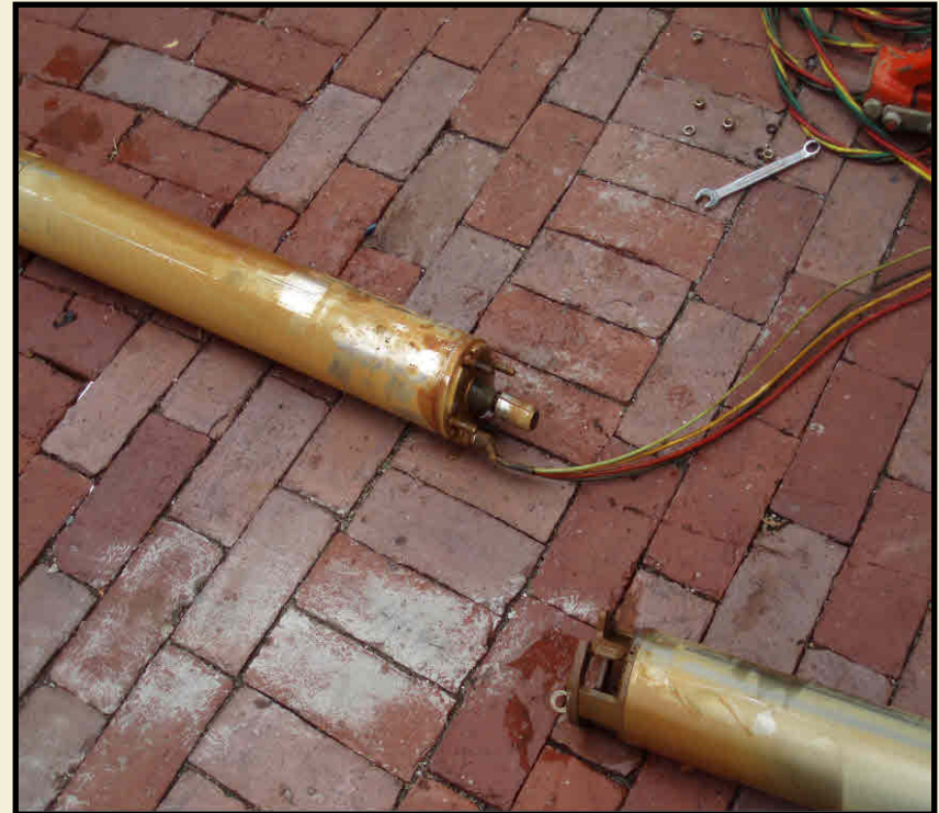
Well Pump Damaged from Low Flow Conditions
