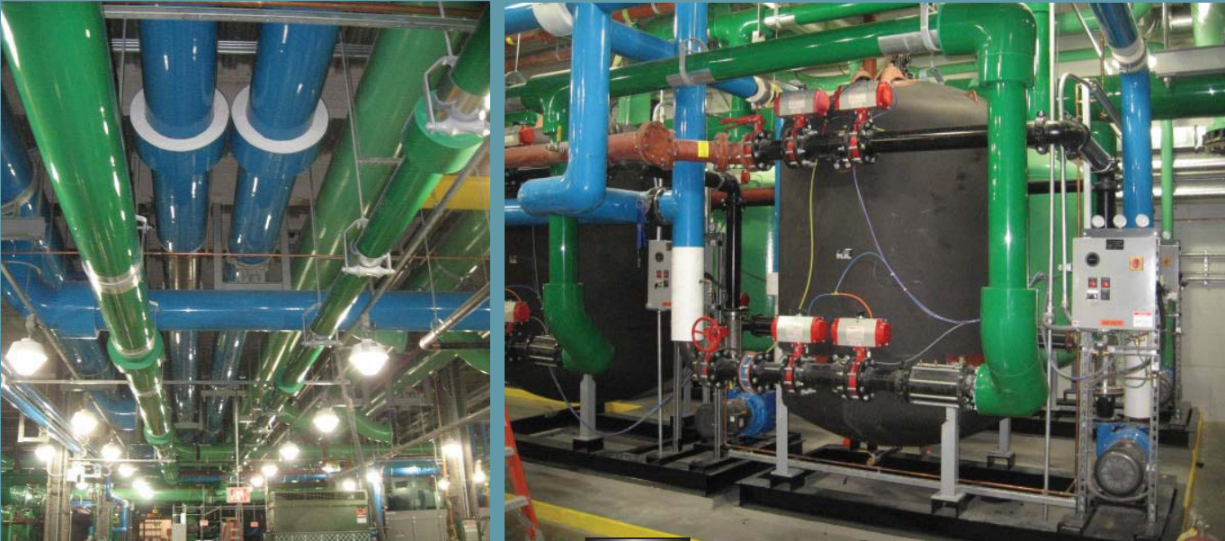
Cooling for 75 University buildings
